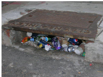
Storm Drain Polluted After Rainfall
