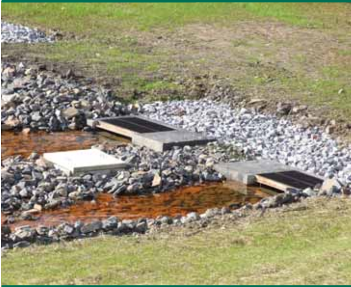
Passive AMD treatment system
